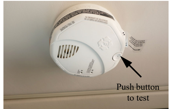
Smoke/carbon monoxide alarm. -Typical View
