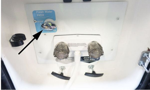
Fresh Water Valve (Located on Water Center Panel shown in normal position). -Typical View
