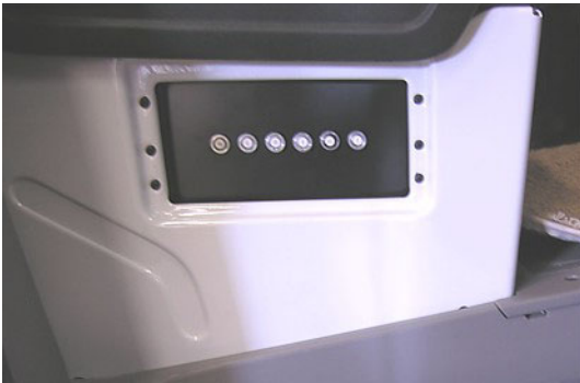
Automotive Chassis 12-Volt Circuit Breakers Located on outboard side of passenger seat (Shown with cover removed). -Typical View
