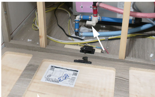
Winterization Valve #1 Water Heater Bypass (Shown in Normal position). -Typical View
