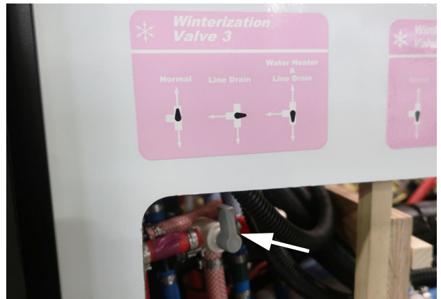
Winterization Valve #3 (Located on Water Center Panel shown in normal position). -Typical View
